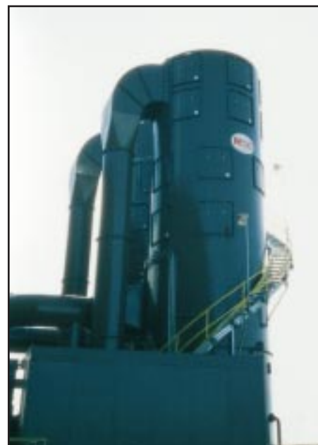
RIGHT Fugitive coal dust collection at a coal-fired utility company.
